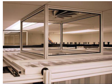
Cold aisle containment with above rack supply air diffuser
