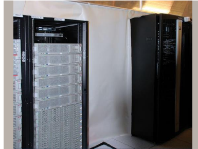
Solution installed to enable easy removal and insertion of racks
